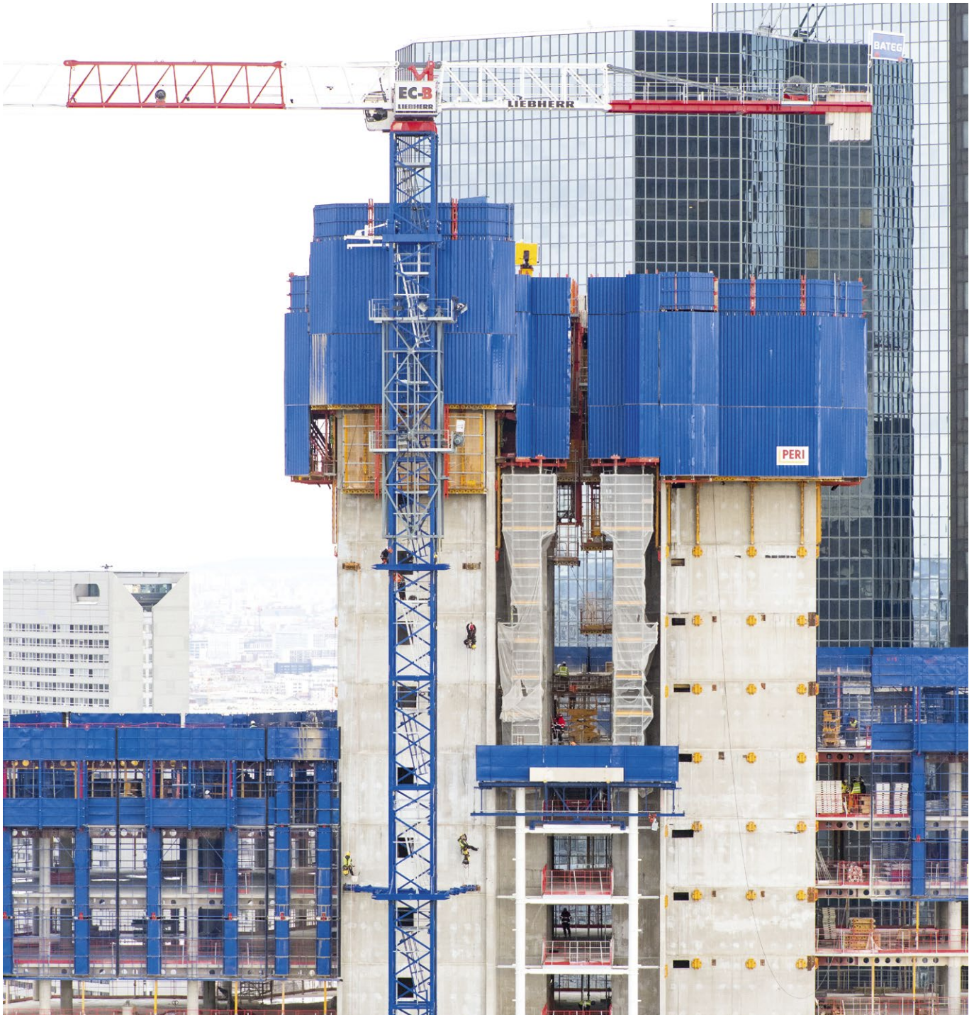
Building construction, Paris la Défense, France © 2019 - Petzl Distribution - Lafouche - Integral - Bateg - Tour Trinity - Cro&Co Architecture
