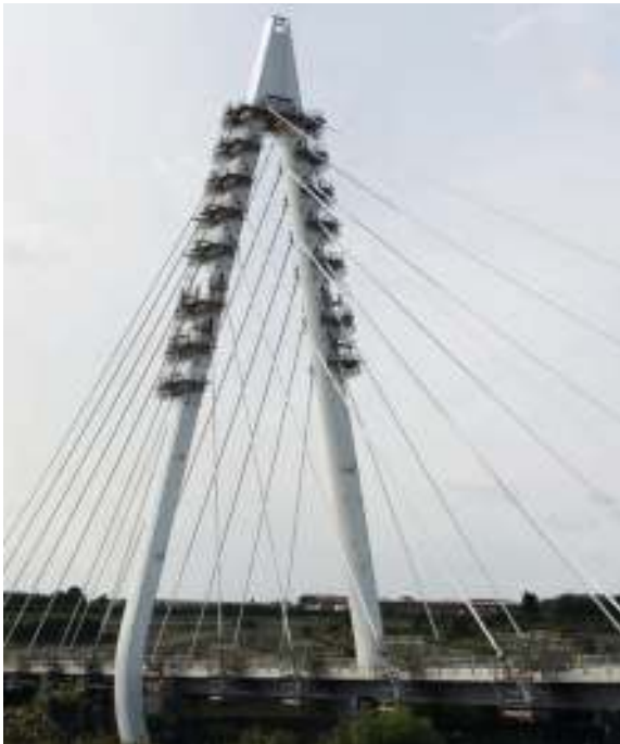
Supplier of access scaffolding to Victor Buyck Steel Construction for the New Wear Crossing, Sunderland
