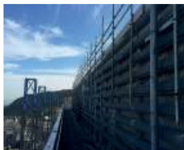
Scaffold in place at Appleton Tower, part of the University of Edinburgh
