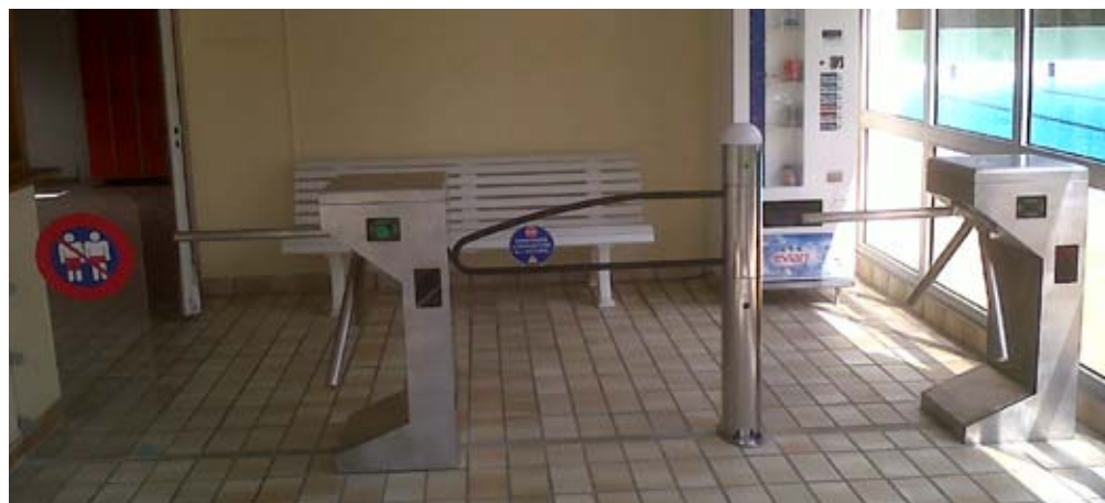
Half Height Turnstile installed at a leisure centre
