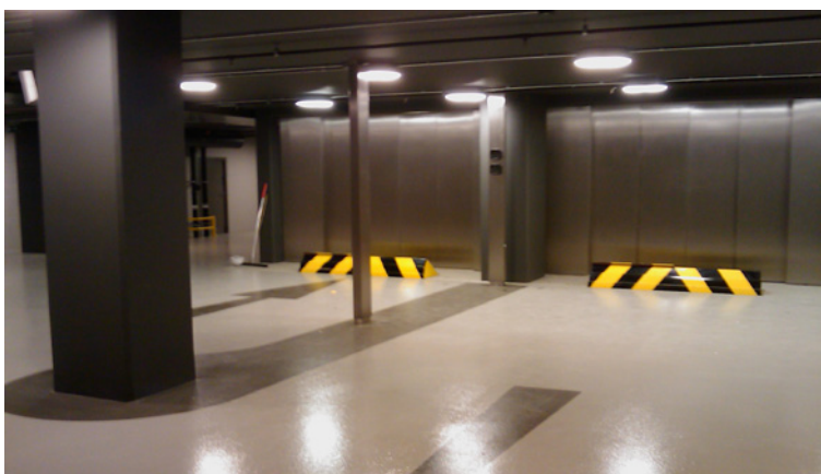
Special Parking Height RoadBlockers installed in front of a vehicle lift of an elite inner city residence
