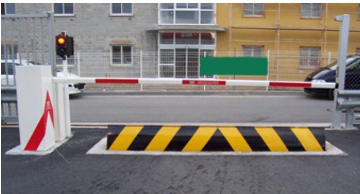
Road blocker's Hydraulic Control Cabinet installed behind an automatic barrier cabinet.
