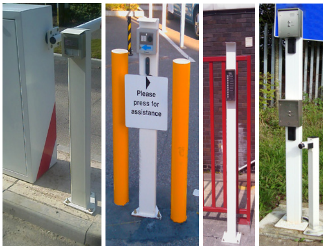
Standard Car Height Pedestals. Installed with bollards for protection
