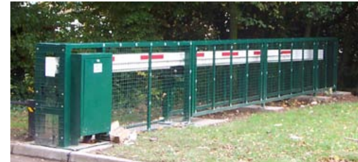
Runback of Barricade Beam fully encased in pedestrian guard rail to ensure no trapping areas.
