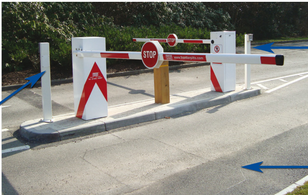
Access Control Pedestal
